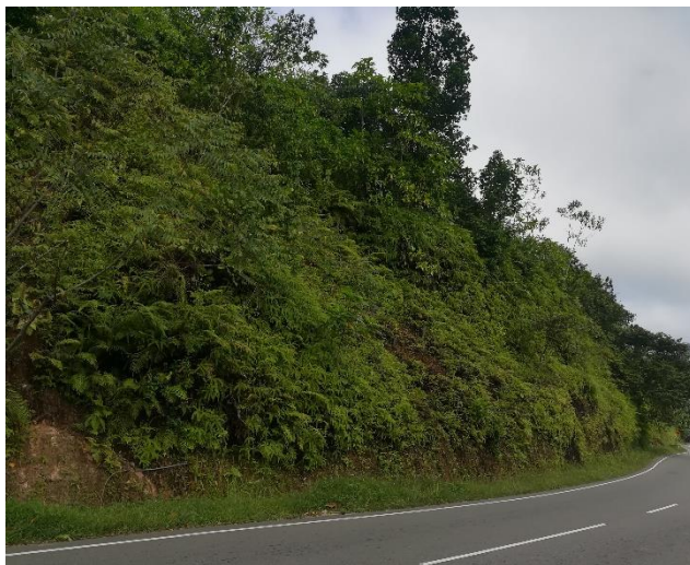
Figure 05 (a) – Natural slope has been altered as the result inappropriate vertical cut for road construction.
